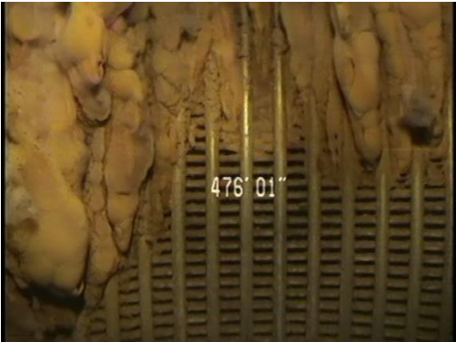
Figure 5. Fouled Well Screen
